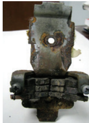
Fig 28: Circuit breaker corrosion
