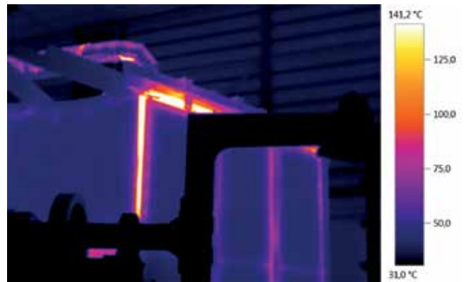
Industrial kiln with faulty insulation.
