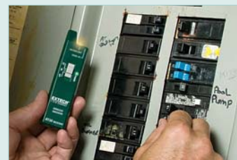
The receiver indicator unit will indicate voltage present. When the user opens the splice or breaker, the voltage present indication stops, thereby identifying the AC wire.
