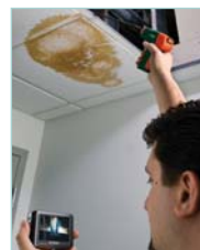
Ideal Applications: - Water Restoration - HVAC and Refrigeration - Electrical inspection - Automotive - Pest control
