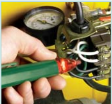
Control panel troubleshoot
