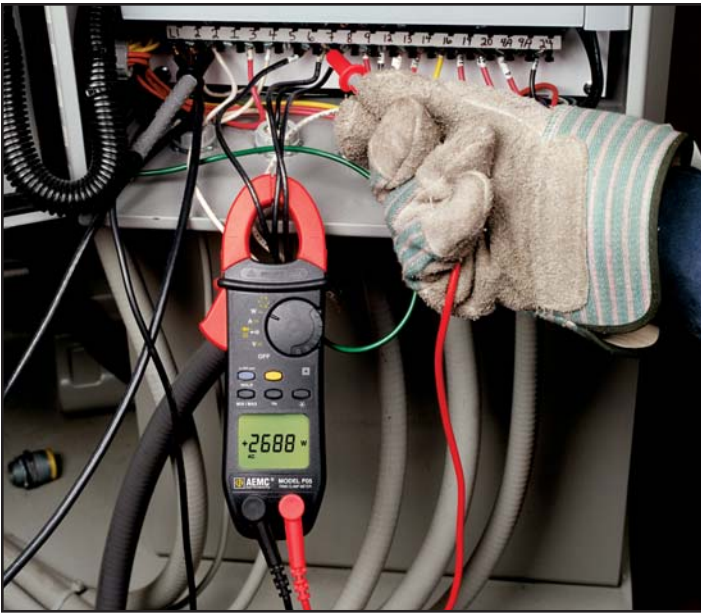
Model F05 monitoring volts, amps and watts on a control panel.
