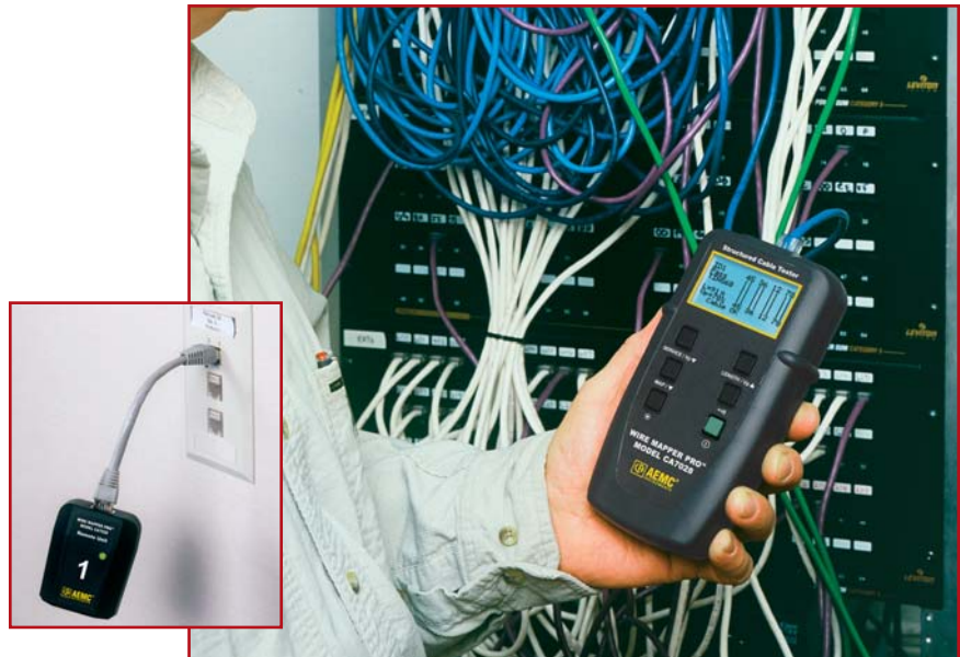
Model CA7028 used to locate and test a cable from the patch panel to an office a few hundred feet away.
