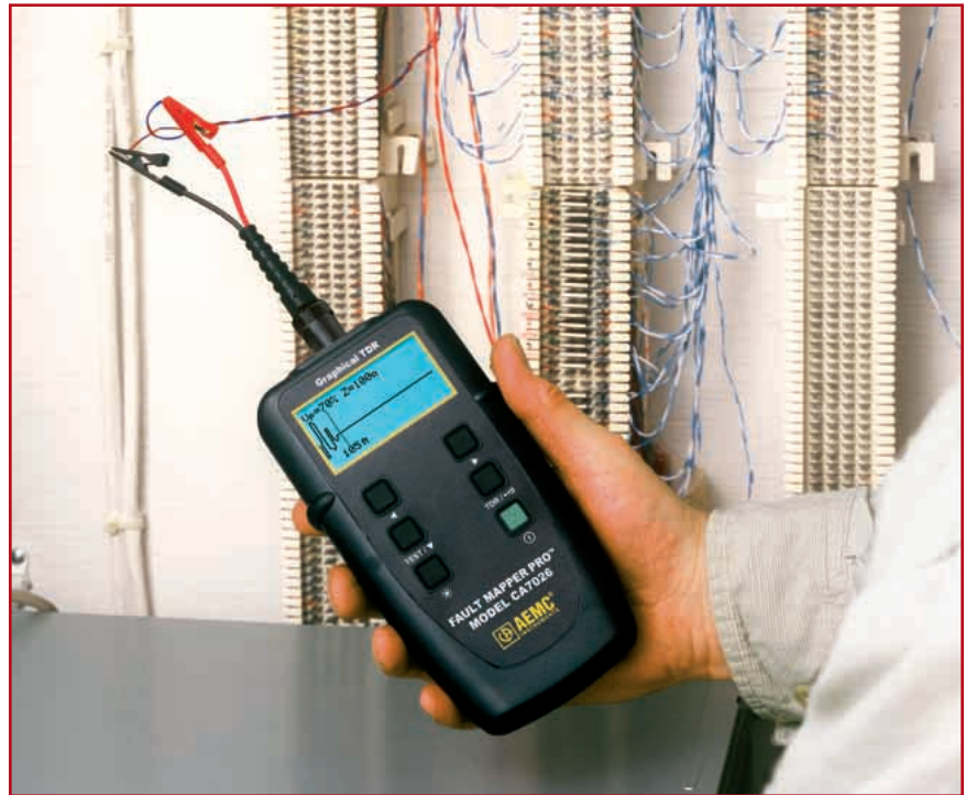
Model CA7026 testing cables in a telephone patch panel.
