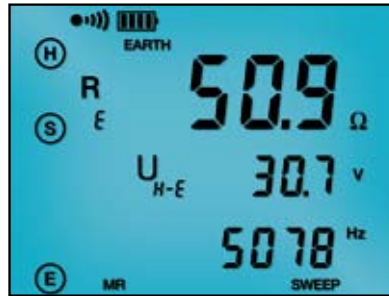
The 3-Point Fall-of-Potential test displaying test lead connection, grounding electrode resistance, test voltage and frequency.
