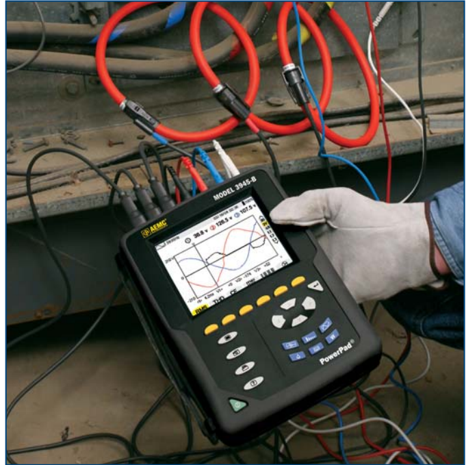
Power quality analysis on a three-phase panel using the AmpFlex ® flexible current probes.
